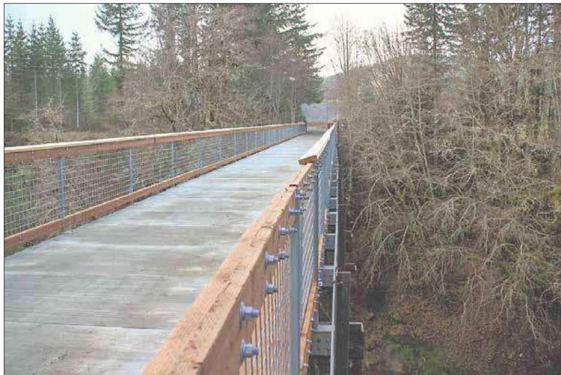
This photo of the recently completed bridge was taken by Chris Brewer and posted to the Ride the Willapa Facebook page.
